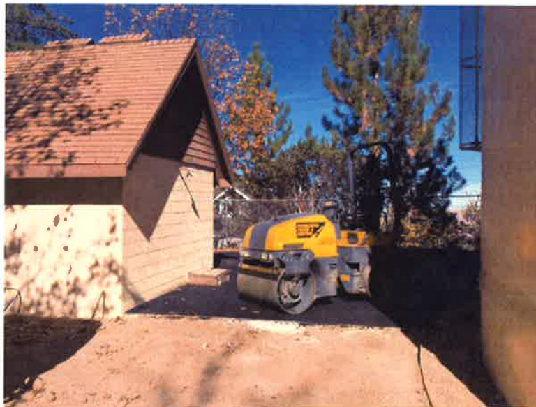
Banff Tank Site
